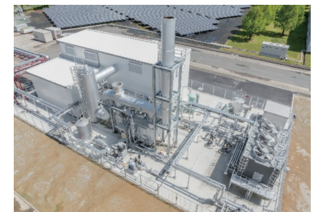
Gas cogeneration system
